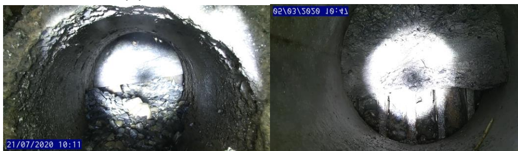
Examples of blocked pipes
